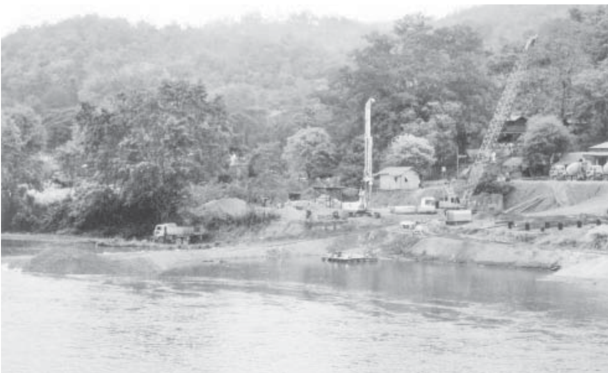
Construction site for building new Hsipaw Dokhtawady Bridge seen in the first week of June.
