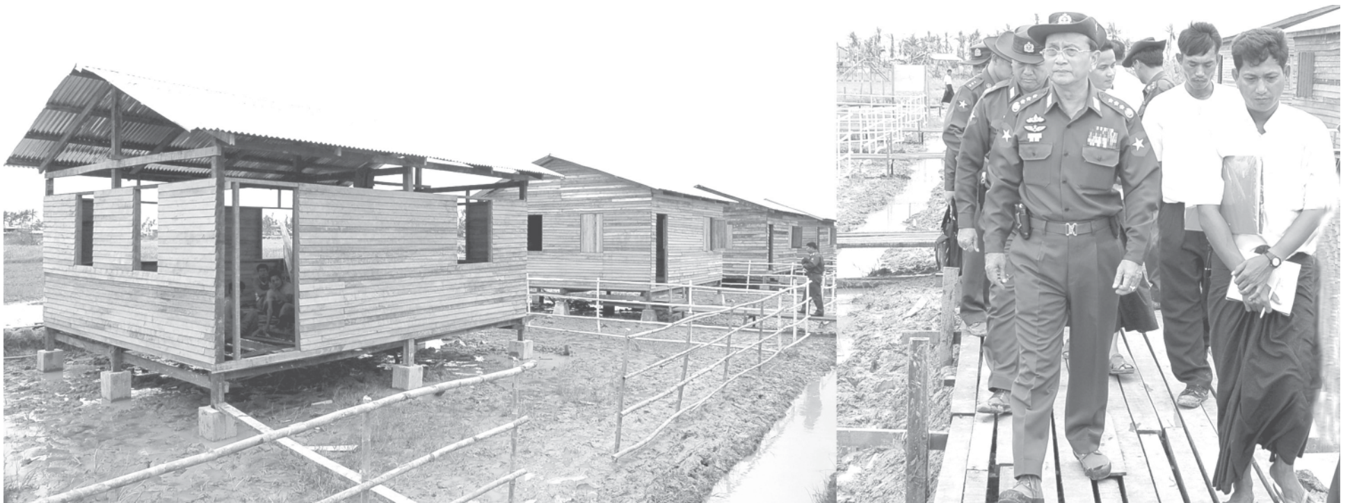
Chairman of NDPCC Prime Minister General Thein Sein views construction of houses by Original Group Co for storm victims in Hlaingbone Village.—MNA
