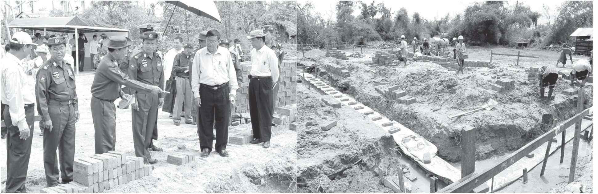
Prime Minister General Thein Sein inspects laying foundation for construction of a school in Dedanaw Model Village.—MNA
