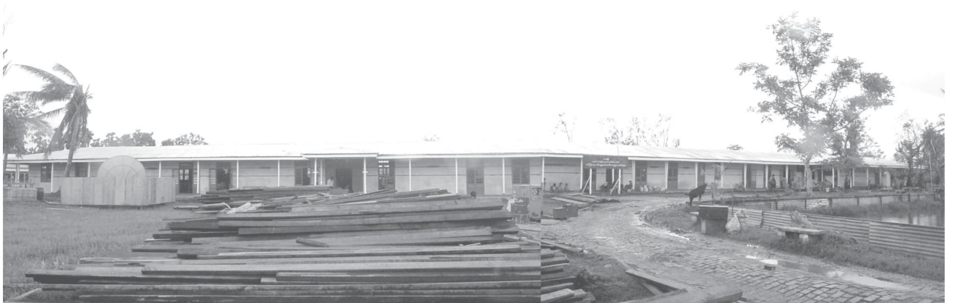
No. 1 Basic Education High School seen after being repaired in Dedaye Township. — MNA
