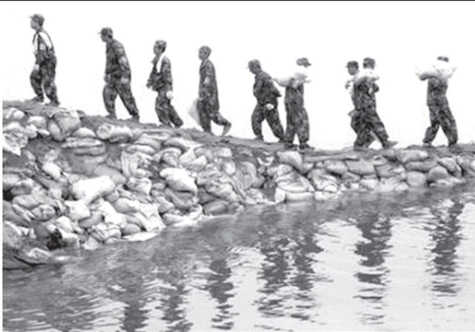
Soldiers build a temporary dam against possible flooding at Quhe River in Suining, Sichuan Province, on 11 June, 2008.—INTERNET
