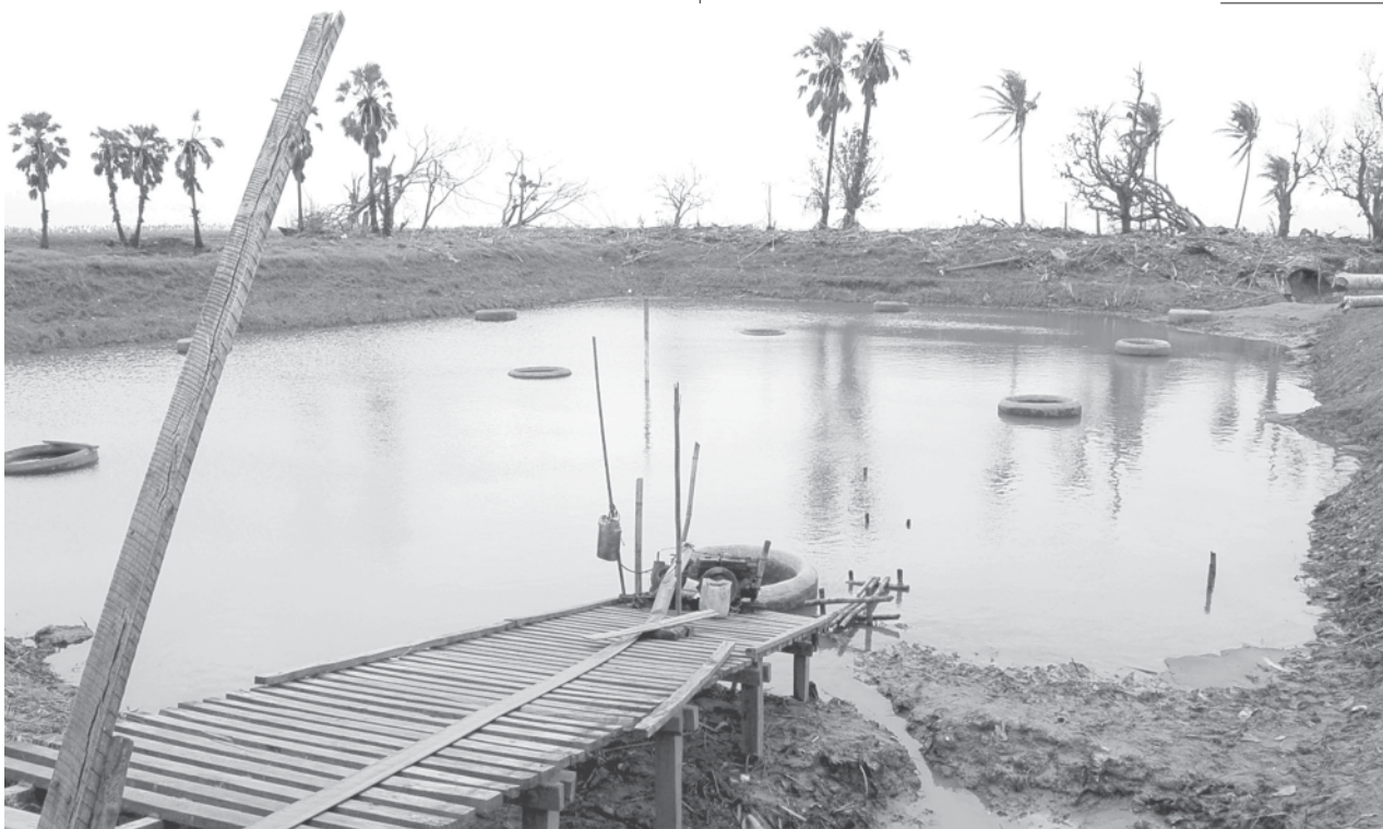
Progress on repair of a lake into which seawater entered in Saluseik village, Labutta Township.—MNA
