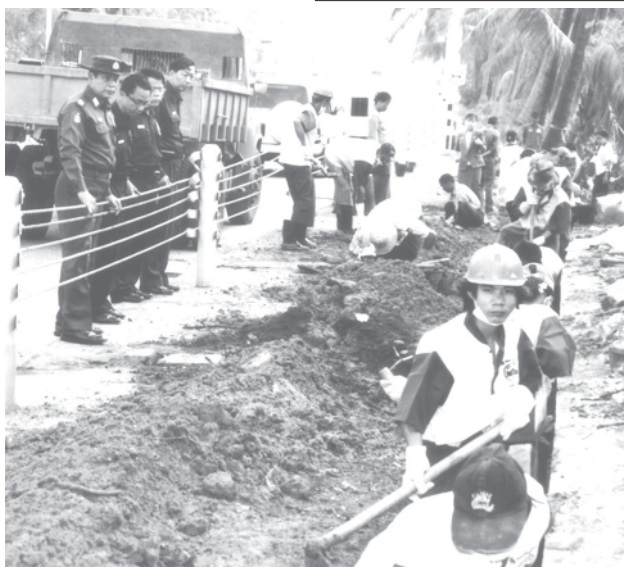
Mayor Brig-Gen Aung Thein Lin inspects dredging of drains near junction of Parami and Pyay roads.—MNA
