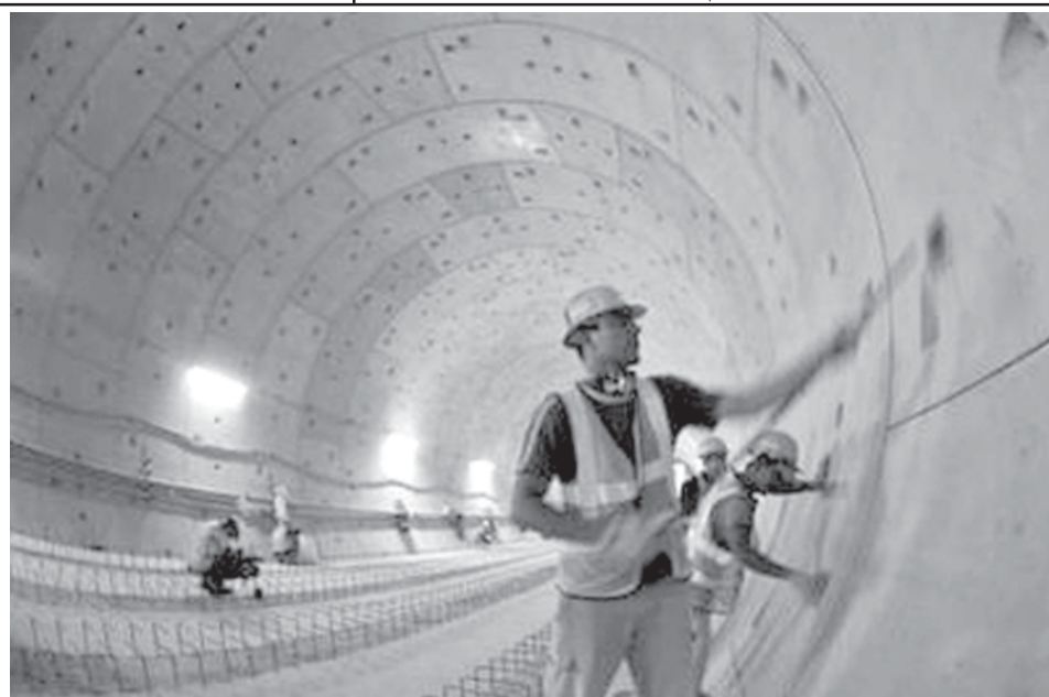
A labourer works in the underground tunnel of Union Square Station, one of two underground stations where both lines meet at Metro Dubai, currently under construction, on 28 May, 2008.—INTERNET
