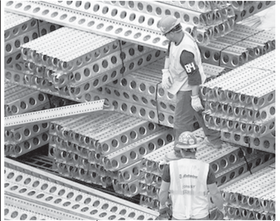
A construction worker stacks steel forms for the Freedom Tower on 19 May, 2008 in New York. Inflation at the wholesale level slowed in April following a huge increase in March although prices for a number of items from prescription drugs to pasta shot upward.—INTERNET
