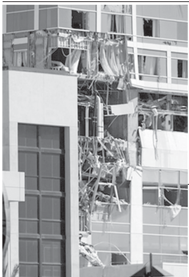
Debris hangs from a damaged section of the Hilton Hotel under construction where an explosion ripped through the floors on 19 May, 2008 in San Diego.
