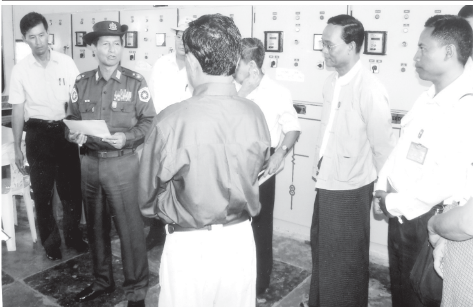
Minister Maj-Gen Khin Maung Myint inspects sub-power station at No 1 Industrial Zone in Shwepyitha.—EP 2
