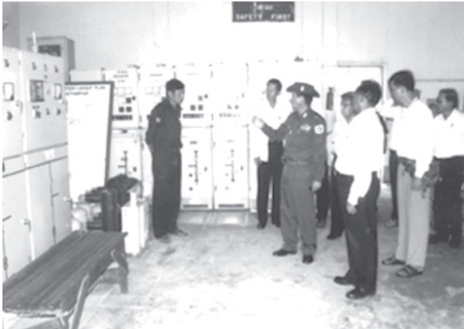
Minister Maj-Gen Khin Maung Myint visits sub-power station No 1 in Hlinethaya Township.—MNA
