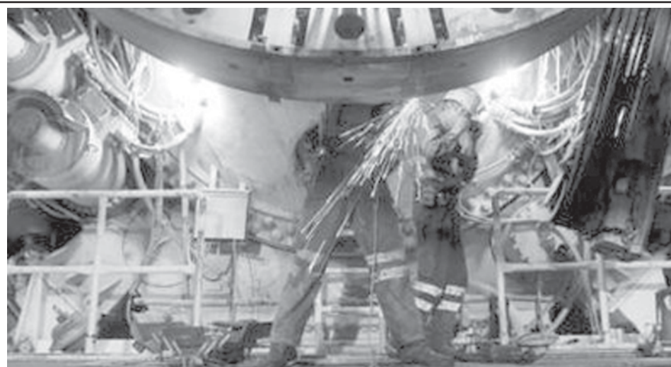
Workers operate on a tunnel drilling machine inside the Gotthard base tunnel in Erstfeld, central Switzerland on 15 May, 2008. The Gotthard base tunnel with a planned length of 57 km (35 miles) which is part of the pan European high speed rail lines, should become operational at the end of 2016 and will be the world's longest railway tunnel.—INTERNET
