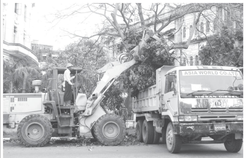
Servicemen of Defence Services Martial Art and Sports Institute take part in clearance of debris along the roads in Kyauktada Township. —MNA
