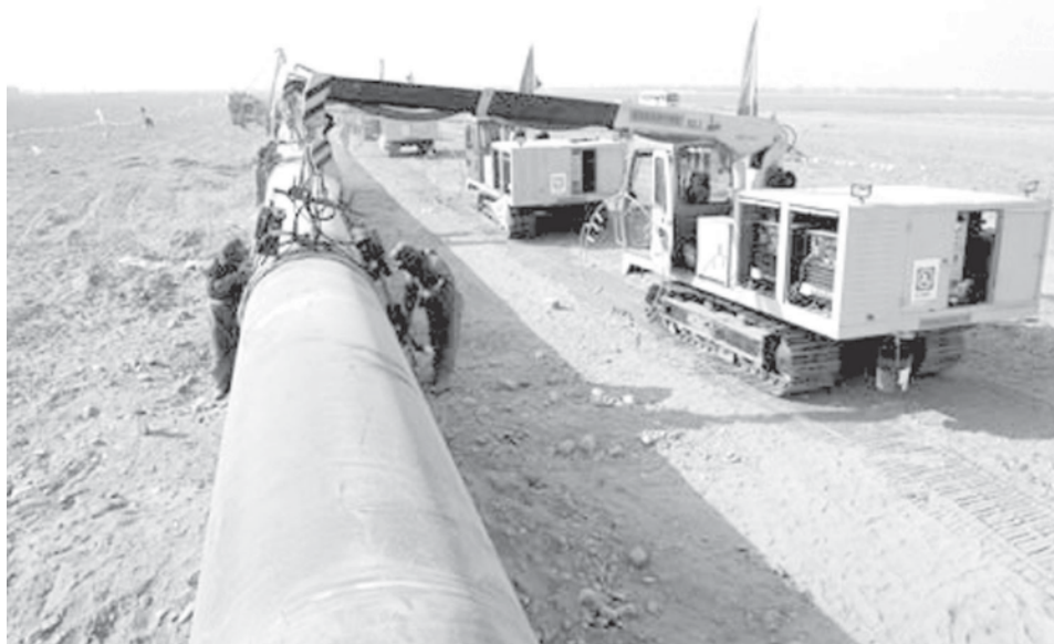
Photo taken on 10 March, 2008 shows the construction site of the second project of west-to-east natural gas transmission pipeline in Fangle Town of Wuwei City, northwest China's Gansu Province. The pipeline will carry natural gas from Turkmenistan and China's Xinjiang Uygur Autonomous Region to the central and west China's areas as well as the Yangtze and Pearl River deltas. — XINHUA
