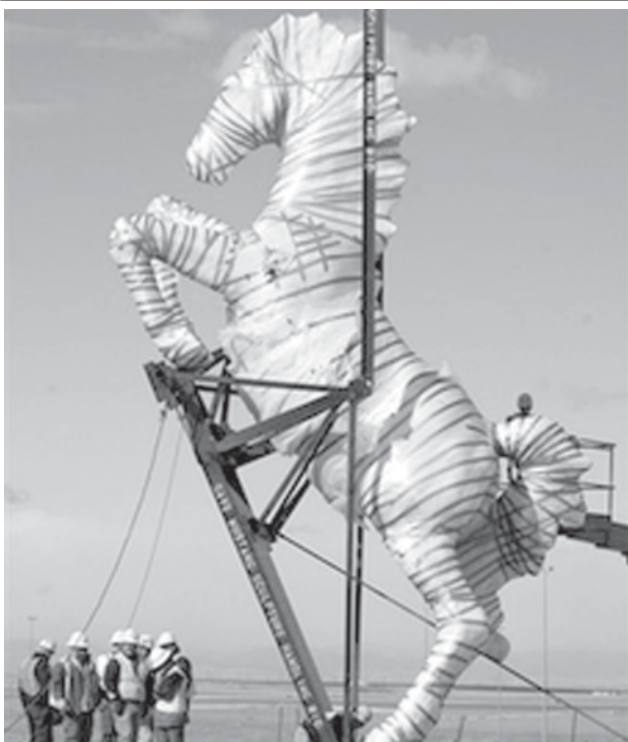
Construction workers install a mustang sculpture at Denver International Airport on 11 Feb, 2008.
