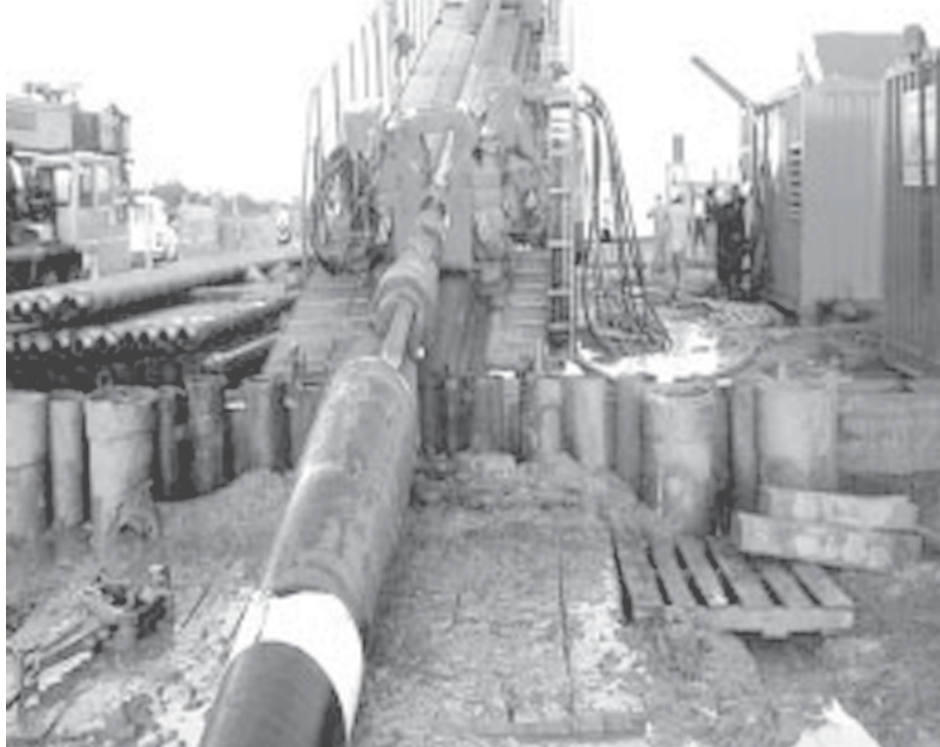
Laying of Myainggale-Yangon natural gas pipelines in progress in Hpa-an District of Kayin State.
