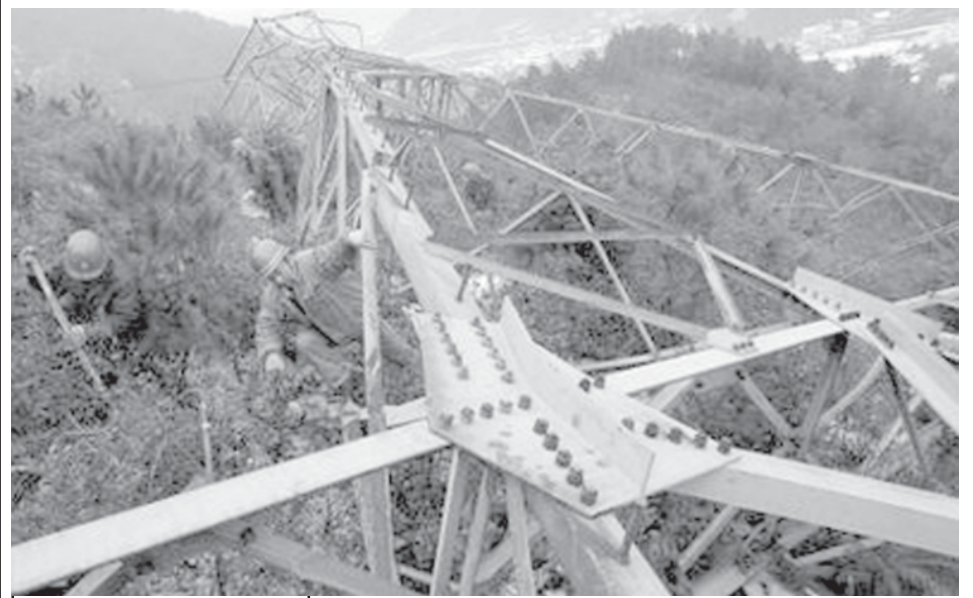
Workers check a power supply tower which had collapsed during heavy snowfall in Wuhan, Hubei Province, on 5 Feb, 2008. INTERNET
