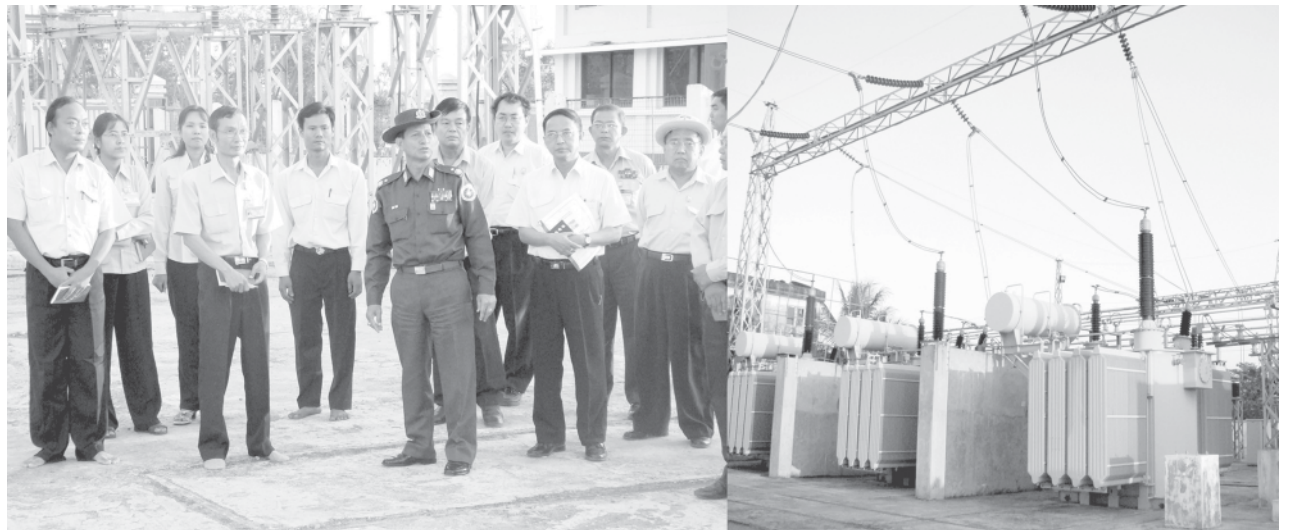
Minister Maj-Gen Khin Maung Myint inspects Bayintnaung Sub-power Station in Mayangon Township. — ELECTRIC POWER NO 2
