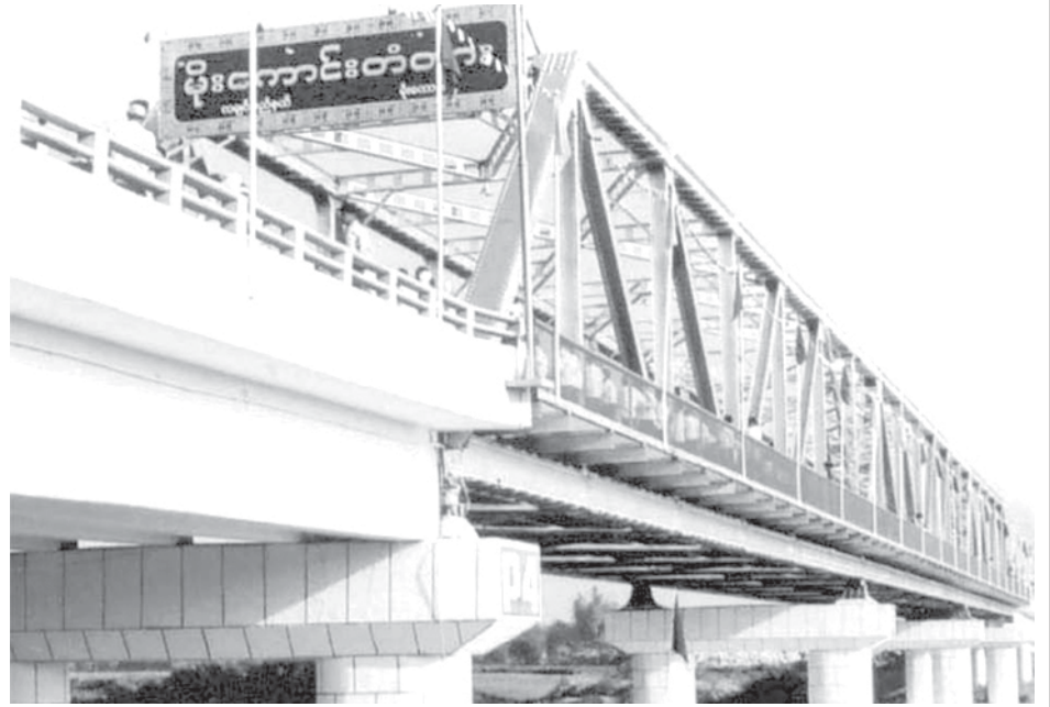
Mogaung bridge in Mogaung Township, Myitkyina District, Kachin State, contributes much to smooth transportation of the region.
