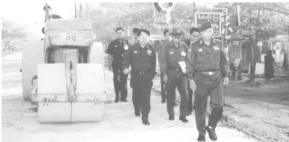
Mayor Brig-Gen Aung Thein Lin inspects paving of Hlawga Road in Dagon Myothit (South) Township. — MNA
