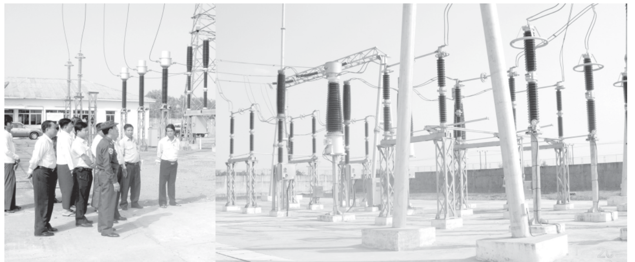
Minister Maj-Gen Khin Maung Myint inspects Myaungdag Power Station in Hmawby Township. — MNA
