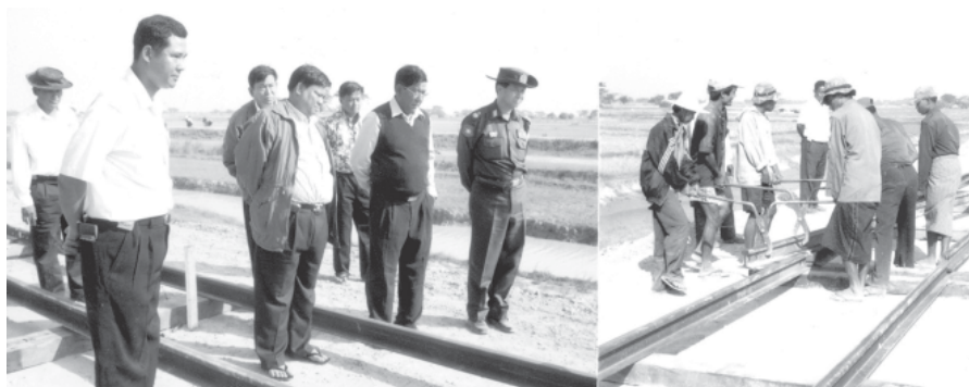
Rail Transportation Minister Maj-Gen Aung Min inspects construction of railroad linking Sittoung and DaikU. — MNA
