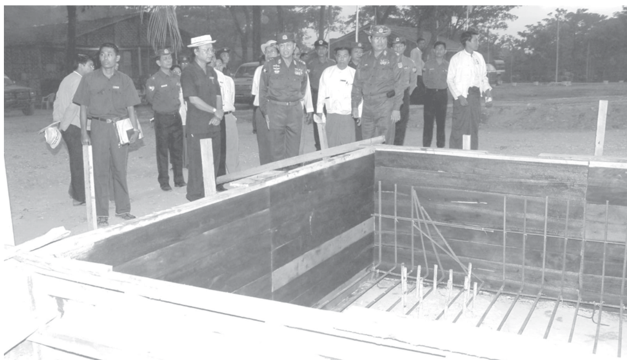
Lt-Gen Khin Maung Than of the Ministry of Defence inspects progress in building Kangyi Bridge on Labutta-Myaungmya-Einme-Kyaunggon-Kyonpyaw road section in Myaungmya, Ayeyawady Division. —MNA
