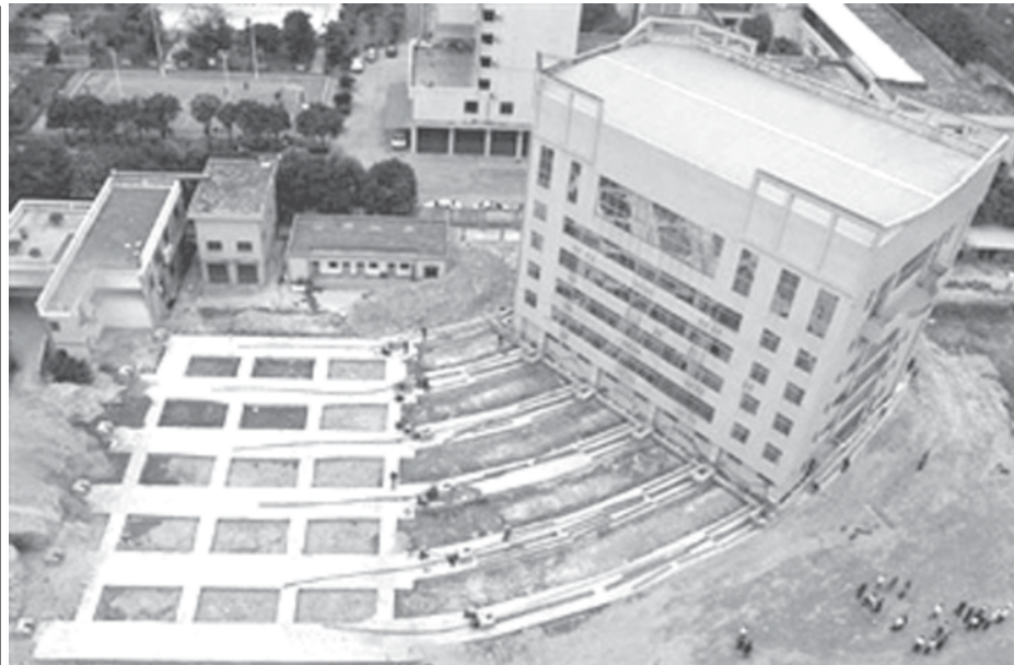
A 5000-ton building is pulled by jacks to its new location in Xiamen, east China's Fujian Province, on 16 Nov, 2006. The building was moved a total of 61 meters (200 feet) from its original position, including a rotation of 45 degrees, China Daily reported.—INTERNET
