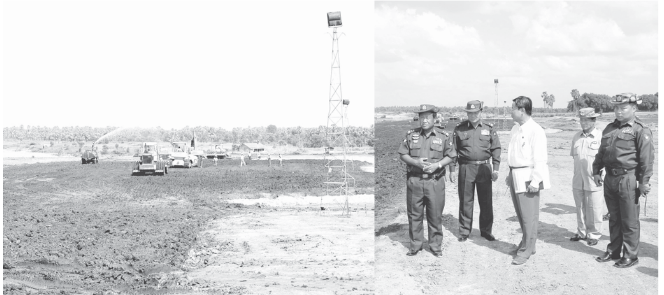
Lt-Gen Ye Myint of the Ministry of Defence inspects Shanmange Dam construction project. — MNA
