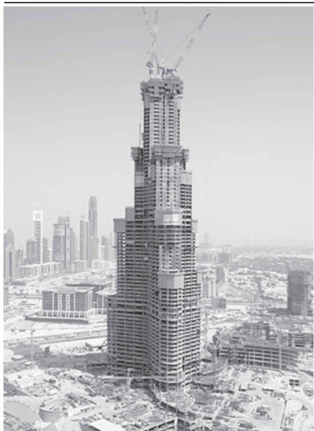
Construction continues on the Burj Dubai skyscraper in Dubai, on 29 Oct 2006. Set to be the world's tallest tower on completion in 2008, Burj Dubai has now clocked up 79 floors.—XINHUA
