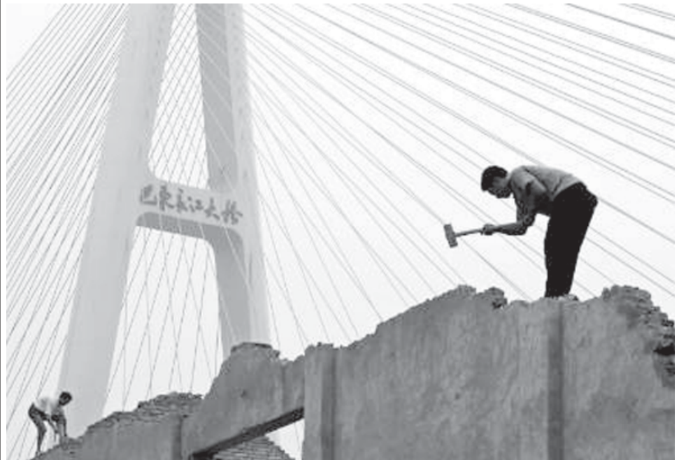
Labourers work to demolish a house near a bridge on the Yangtze River in Enshi, Enshi Tujia Autonomous Prefecture, central China's Hubei Province, on 20 Oct, 2006. —INTERNET
