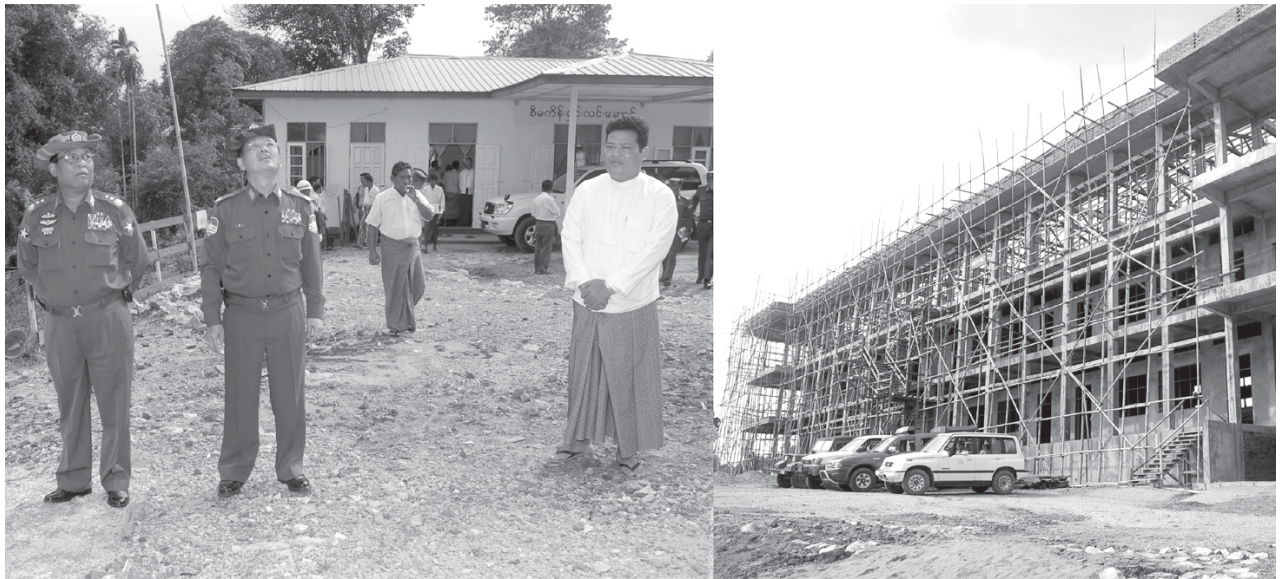
Lt-Gen Maung Bo of Ministry of Defence inspects construction project of Government Technological College (Myeik). — MNA
