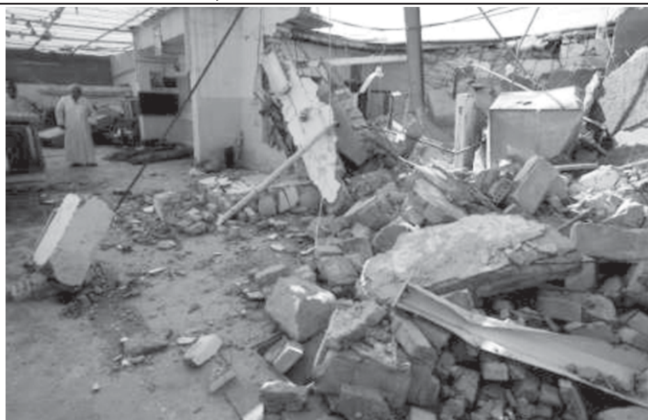
Men stand outside a building damaged after a raid by the US forces in Baghdad, on 20 Oct, 2006. US forces raided the building in the Risala district in southern Baghdad, killing one person and detaining two, police and witnesses said.—INTERNET
