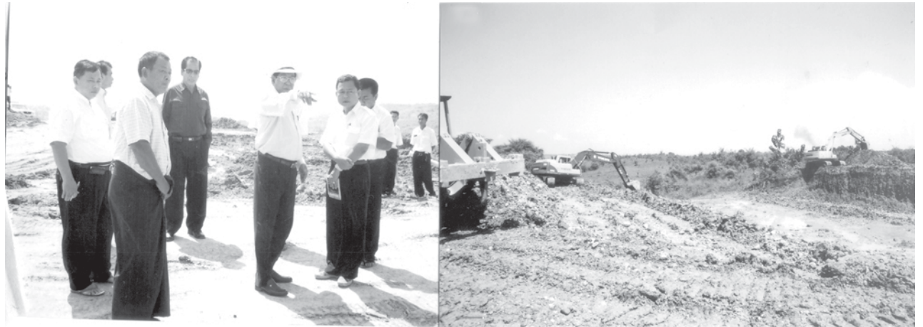
Deputy Minister U Pe Than inspects construction of Kyangin-Okshitpin railroad section. — MR
