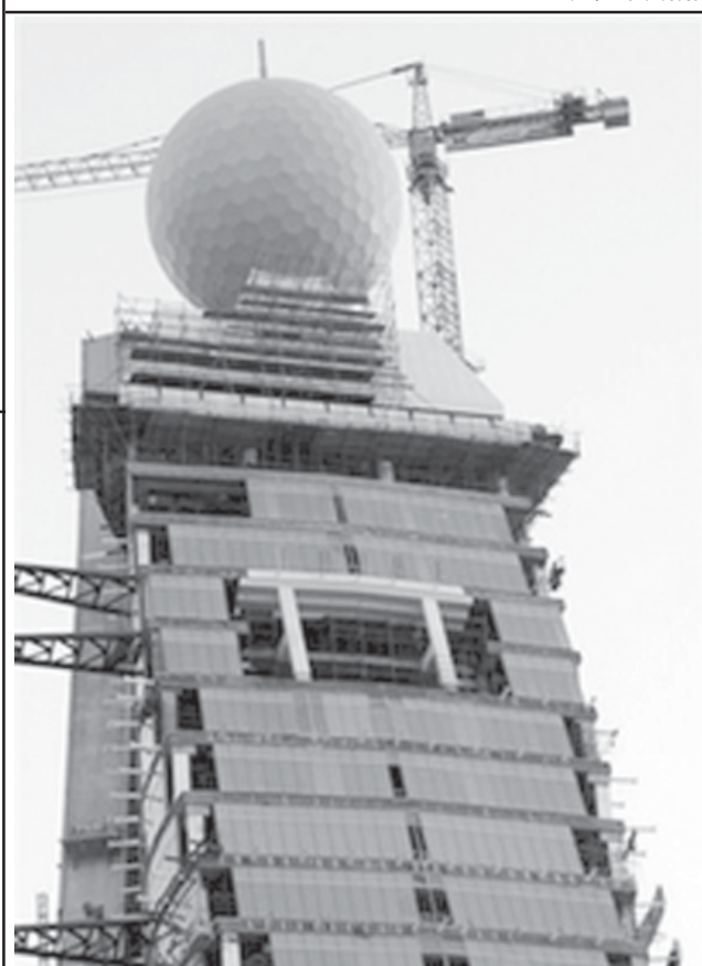
Construction works go on Etisalat new tower on 17 Oct, 2006 in Dubai, United Arab Emirates.
