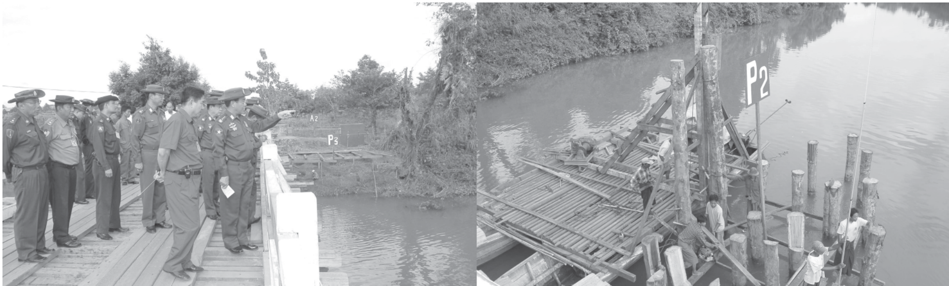
Prime Minister General Soe Win inspects construction of Shweaik Bridge across Nankwe Creek in Myitkyina. — MNA
