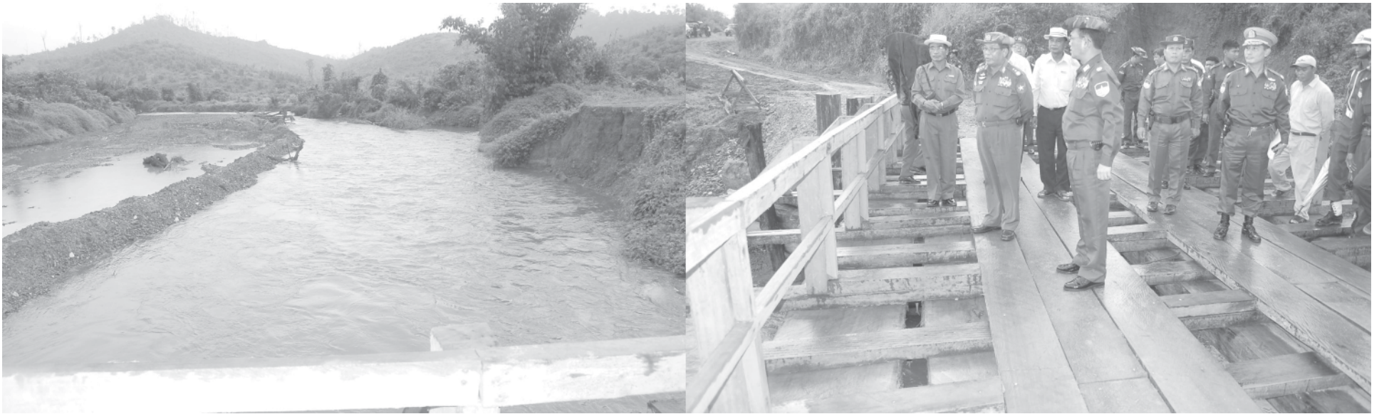
Lt-Gen Maung Bo of the Ministry of Defence inspects renovation of Chaungkabya bridge. — MNA
