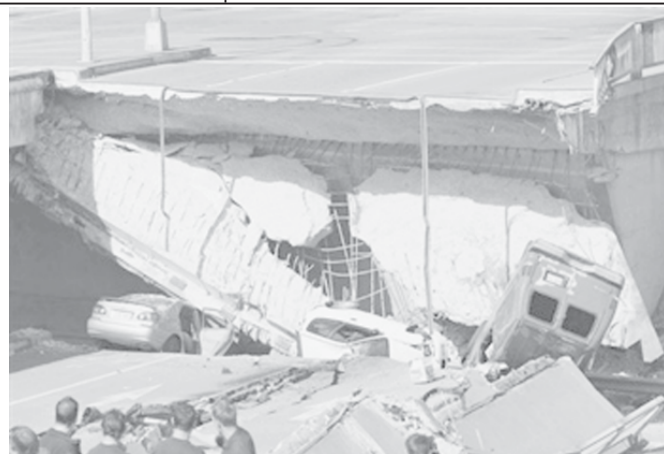
Rescue workers at the scene of a collapsed highway overpass road in the Montreal suburb of Laval, on 30 Sept, 2006. At least five people were taken to hospital on Saturday after the overpass collapsed, emergency officials said.—INTERNET
