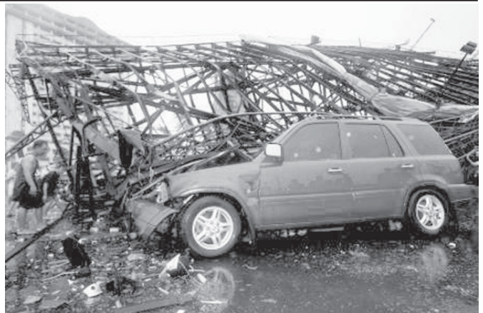
A vehicle is damaged by a billboard structure after the structure was blown down by strong winds of typhoon Xangsane in Manila on 28 Sept, 2006.—INTERNET
