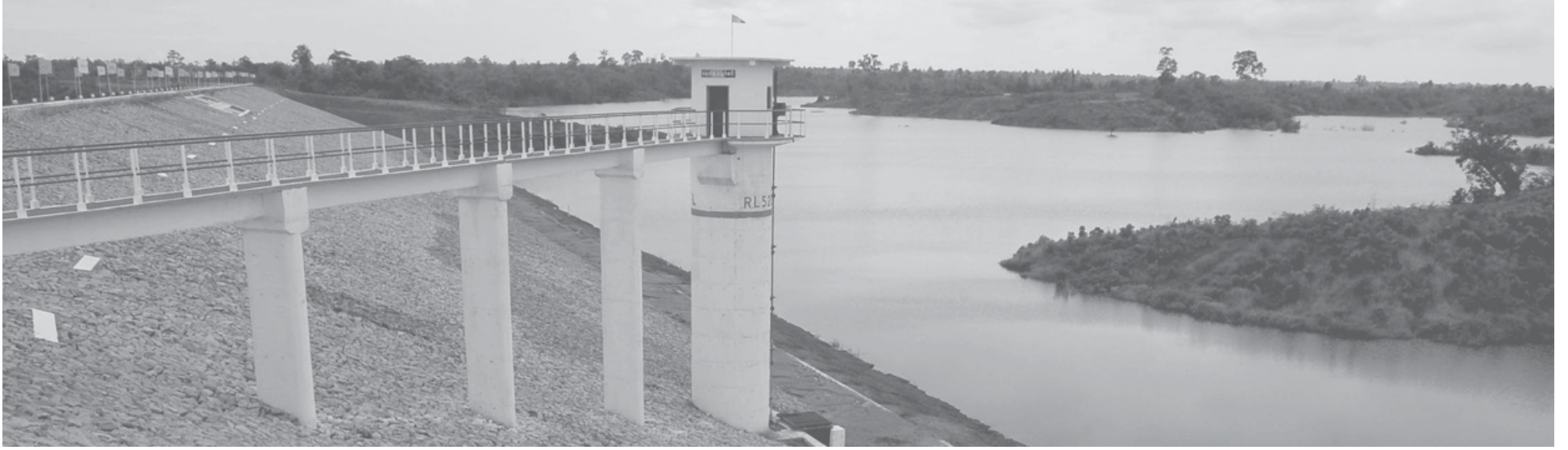
Chaungmange Dam near Pannyosan Village in Lewe Township, Pyinmana District: Chaungmange Dam is of earth embankment. It has 103 square-miles of watershed area. The embankment is 96 feet high and 2,150 feet long. The dam can store 91,770 acre-feet of water. One 50-kilowatt generator will be installed at the dam for producing 0.6 million kilowatt hours yearly. The dam will irrigate 8,000 acres of farmland.
