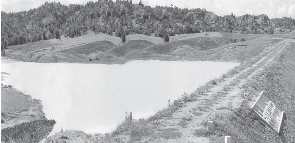
Photo taken on 6 September shows the progress of construction of Po Ni Dam in Seikpyu Township, Pakokku District, Magway Division, for the greening of the region and supply of irrigation water.
