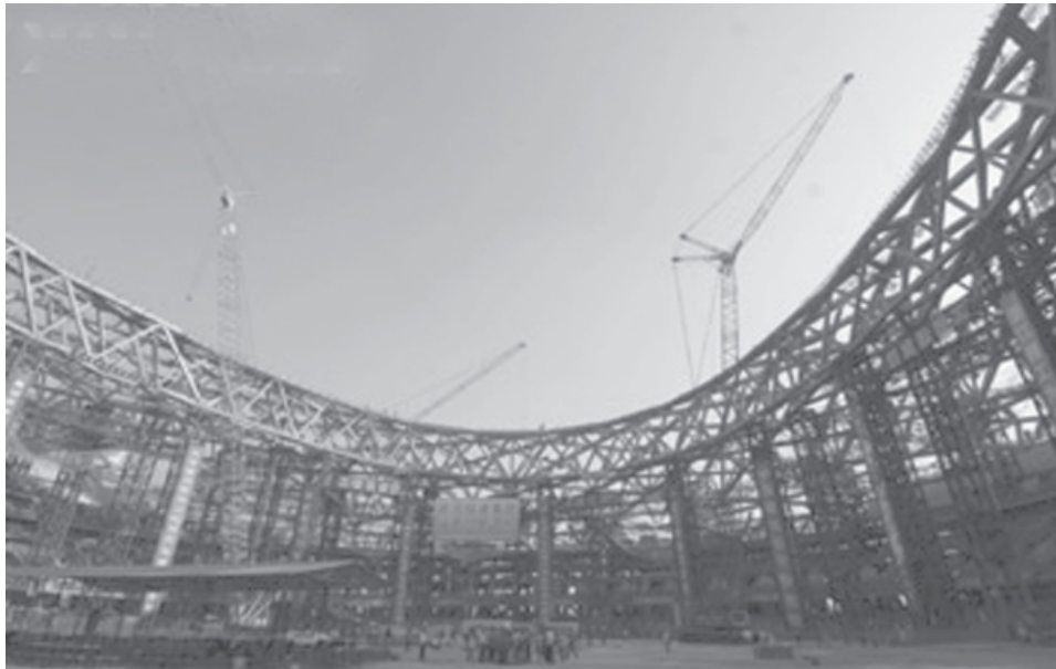
Photo taken on 17 Sept, 2006 shows an inner view of the National Stadium of China. The supporting structure of the National Stadium was successfully removed in Beijing, capital of China, on Sunday. The 91,000-seat National Stadium, known as "Bird's Nest" for its giant latticework structure of metal girders, will host the opening and closing ceremonies and athletics events at the 2008 Games.—XINHUA
