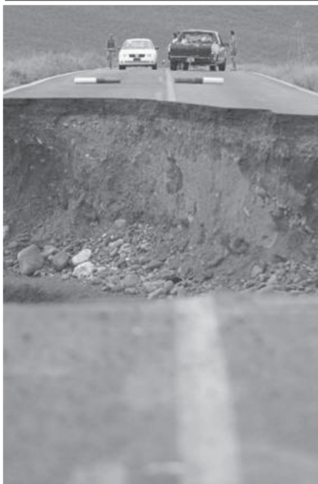
Drivers wait at a damaged road outside of Culiacan in Mexico's state of Sinaloa after Hurricane Lane hit the area on 17 Sept, 2006.—INTERNET
