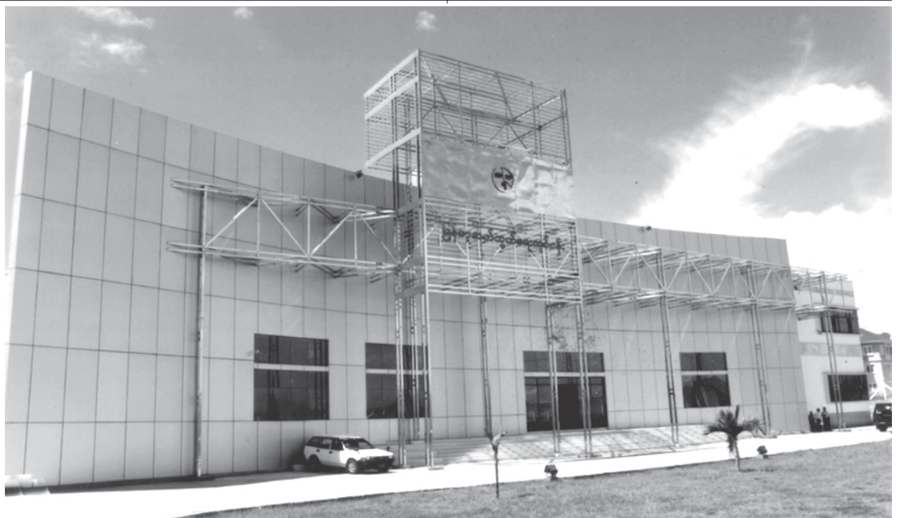
Progress in construction of Nay Pyi Taw Auto-exchange of Myanma Posts and Telecommunications in Nay Pyi Taw. (News reported) — MNA
