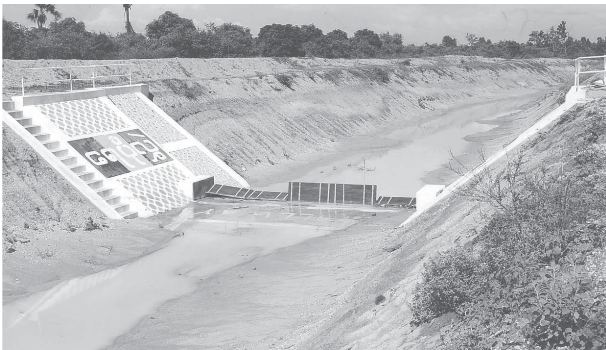
The 25-foot-wide and 3,000-foot-long spillway of Ingyin Thaboe Dam being built in Dabayin Township, Shwebo District, Sagaing Division.
