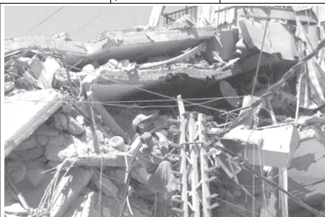
A Lebanese worker fixes electricity cables in front of a building in a southern Beirut suburb that was damaged in the recent conflict between Israel and Hizbollah on 4 Sept, 2006. —INTERNET
