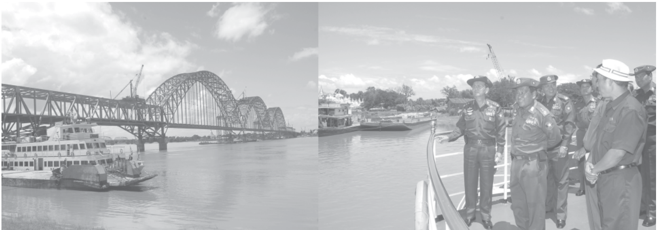
Secretary-1 of the State Peace and Development Council Lt-Gen Thein Sein views progress of Ayeyawady Bridge (Yadanabon) Project. — MNA
