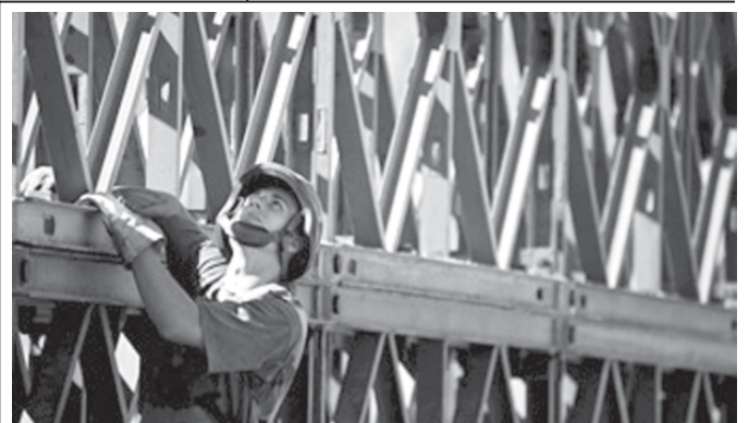
A soldier of the 2nd corps of engineers of the French Foreign Legion works to build a bridge in Damour, south of Beirut, on 3 Sept, 2006. Some two hundred and forty French soldiers arrived in the Lebanese capital on a humanitarian mission to rebuild bridges damaged by Israeli bombing in southern Lebanon.—INTERNET
