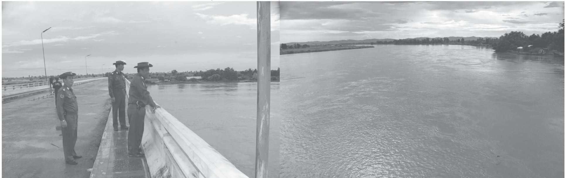
Lt-Gen Ye Myint of Ministry of Defence inspects renovation of Shweli Bridge (NgaO). — MNA
