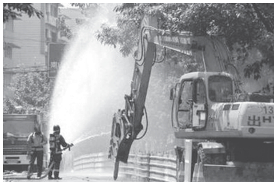
Firefighters use water to control natural gas leaking from a destroyed pipeline on a street in southwest China's Chongqing Municipality on 30 Aug, 2006. More than 200 people were evacuated and gas supply to 170 thousand users was cut off due to this gas leakage.—INTERNET
