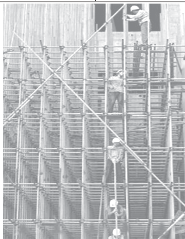
Workers remove scaffolding at a construction site in Shanghai on 23 Aug, 2006, —INTERNET
