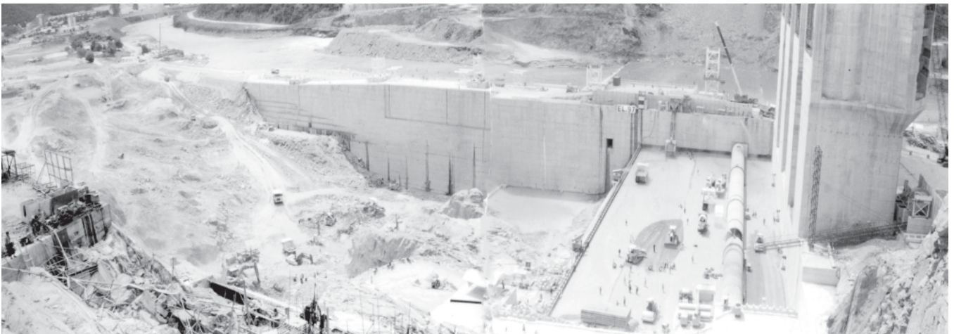
Yeywa Hydrel Power Project. —ELECTRIC POWER No 1
