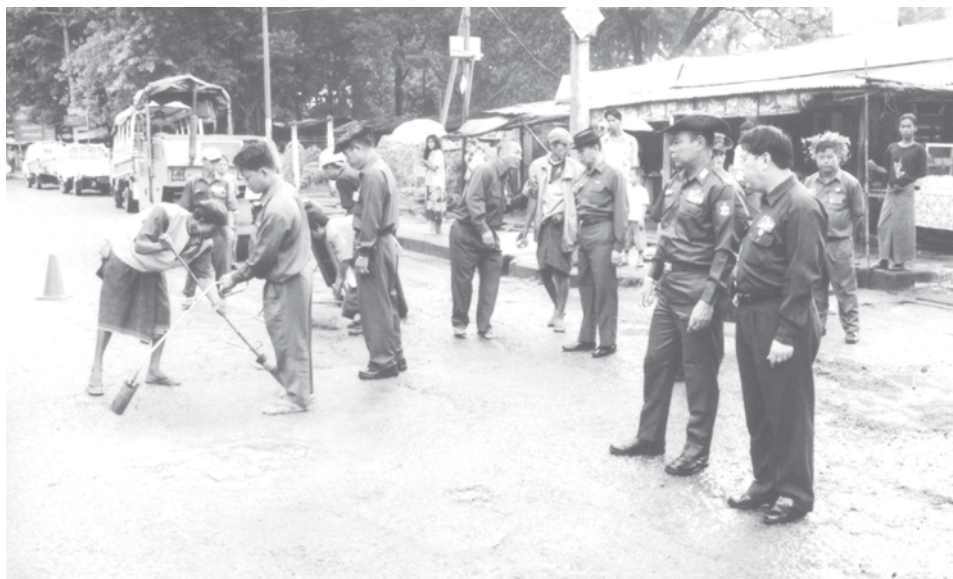
Mayor Brig-Gen Aung Thein Lin inspects repair work on Kyaikkasan Road in Tamway Township. — YCDC
