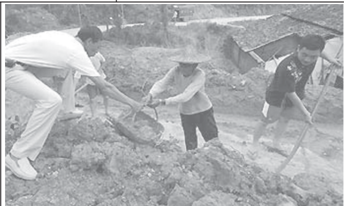
Local people repair a road damaged in floods brought by typhoon Saomai in Huangbo Town of Zherong County, southeast China's Fujian Province, on 13 Aug, 2006. Electricity and communication links are being restored and roads are reopened in some of the disaster areas in Fujian Province as the reconstruction work of the typhoon-hit areas are underway.—INTERNET
