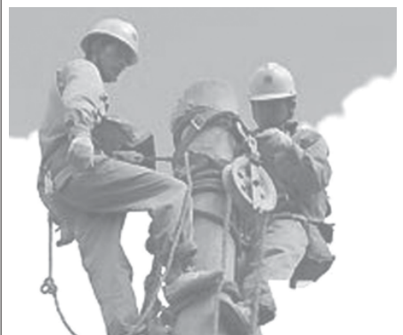
Workers with local electric power department repair electricity system damaged by typhoon Saomai in Zherong County, southeast China's Fujian Province, on 13 Aug, 2006.— INTERNET
