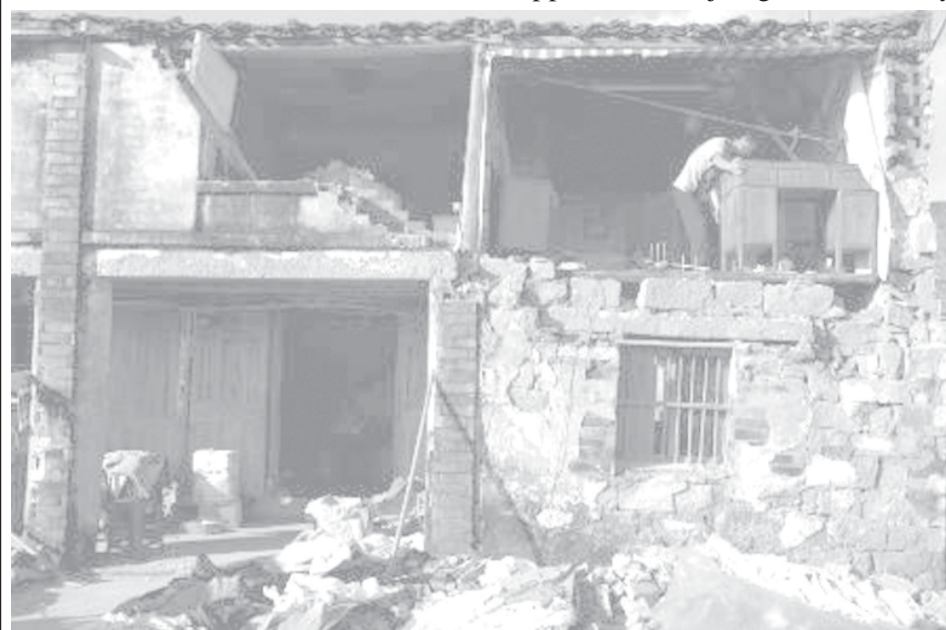
A man attempts to salvage his belongings from a house destroyed by Typhoon Saomai in eastern Province of Zhejiang on 12 August, 2006. Typhoon Saomai punched into Cangnan County on Thursday after authorities had moved hundreds of thousands in the densely populated commercial province to safety. —INTERNET
