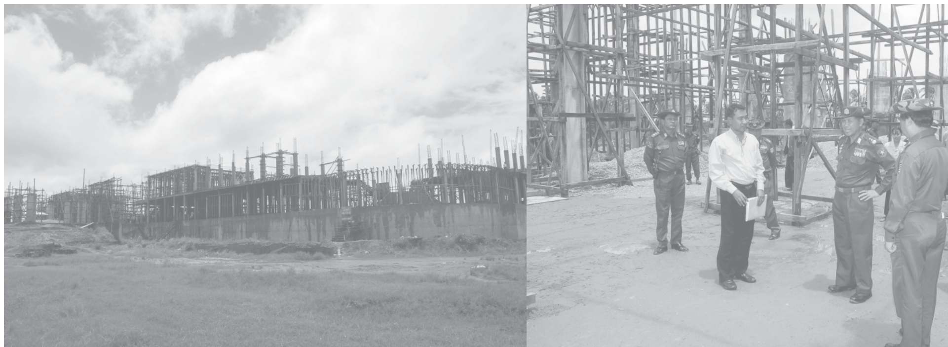
Lt-Gen Khin Maung Than inspects construction of three-storey building of Government Technological College (Hinthada).—MNA
