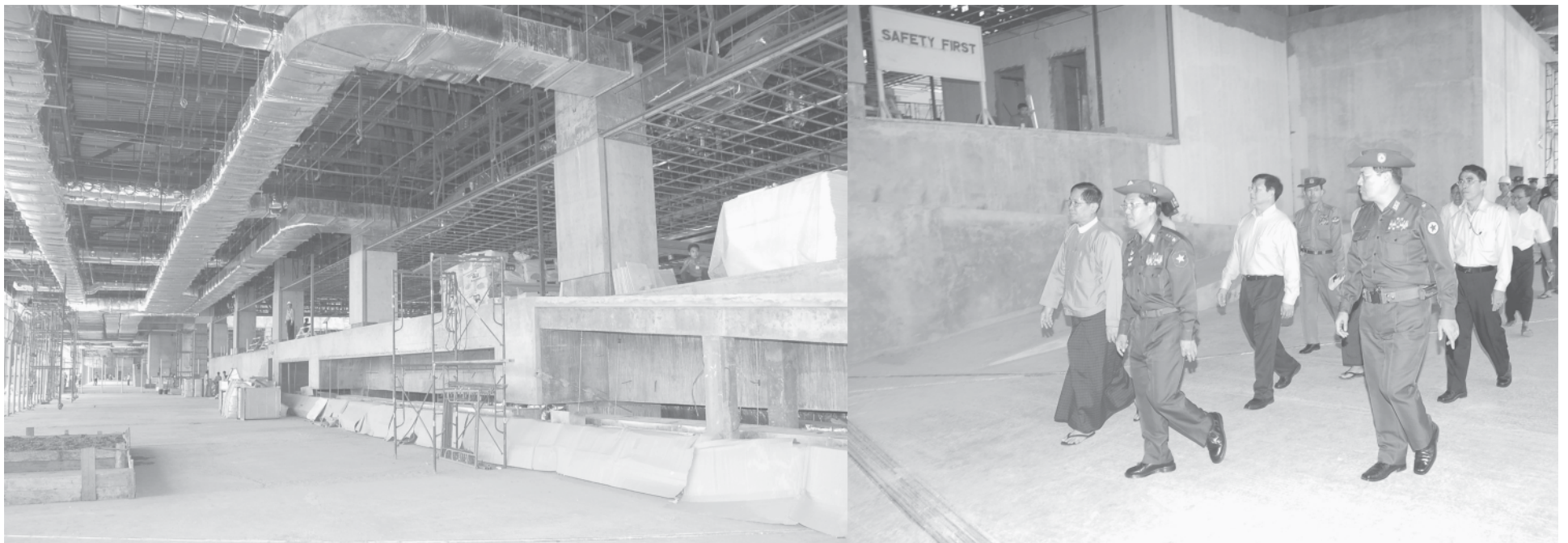
Lt-Gen Myint Swe inspects the tasks for extension of the Yangon International Airport.—MNA
