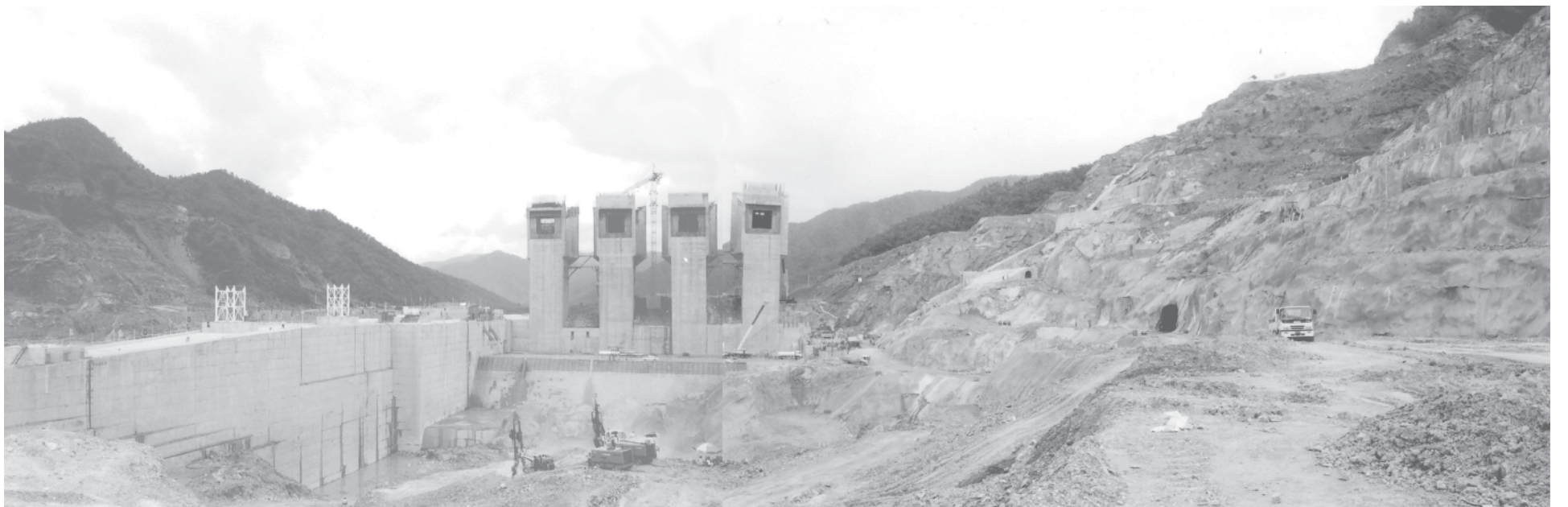
Yeywa Hydel Power Project. — ELECTRIC POWER-1
