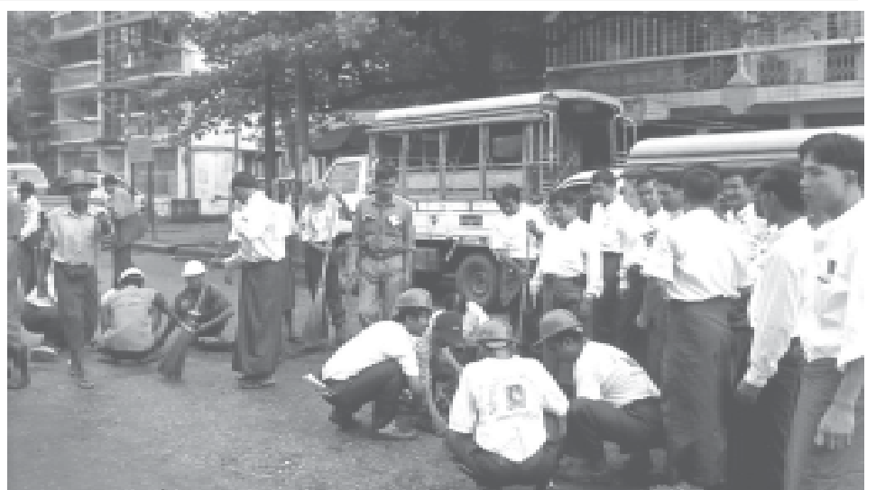
Members of USDA repaving Daw Thein Tin road in Mingalar Taungnyunt Township on 30-7-2006. — MNA
