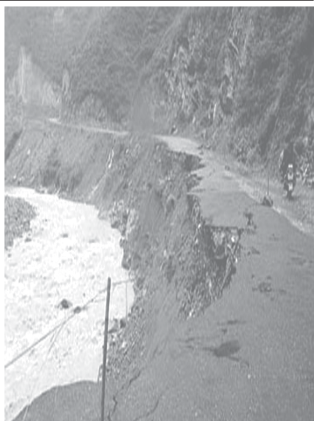
A motorcyclist rides on a flood-damaged road after tropical storm Kaemi, in Shangyou County, East China's Jiangxi Province on 25 July, 2006.—INTERNET
