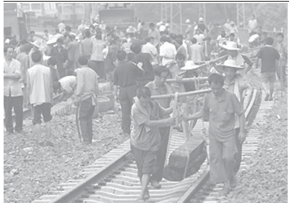
Workers repair a section of railway which was damaged in the earthquake in Yanjin County, Zhaotong City, in the northern area of southwest China's Yunnan Province, on 22 July, 2006.—INTERNET
